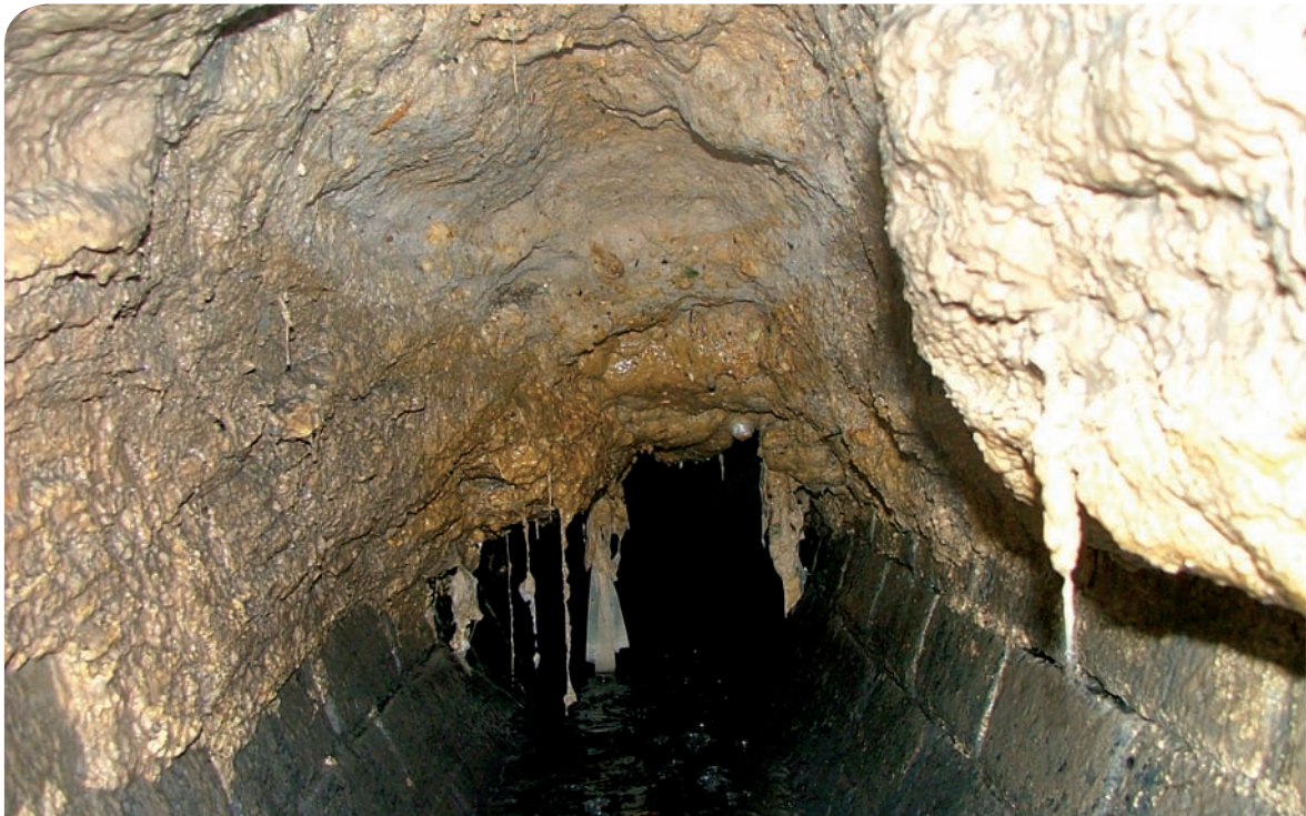
Fat beginning to block a sewer
